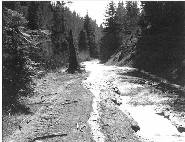
This road has become a drainage channel.
