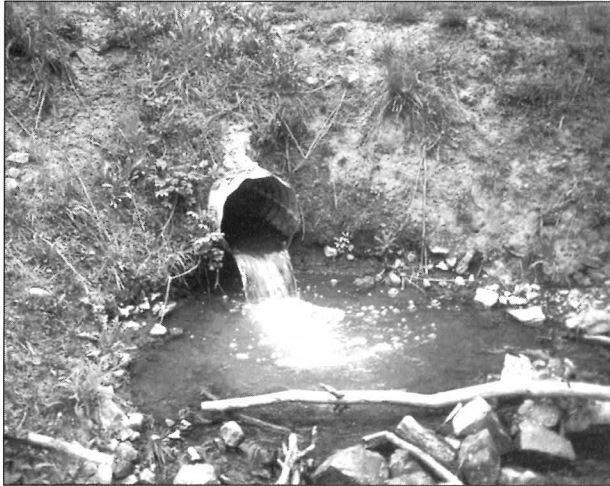
This culvert was too small to carry flood waters and has been replaced. Improperly designed or sized culverts can block miles of upstream spawning and rearing habitat.
