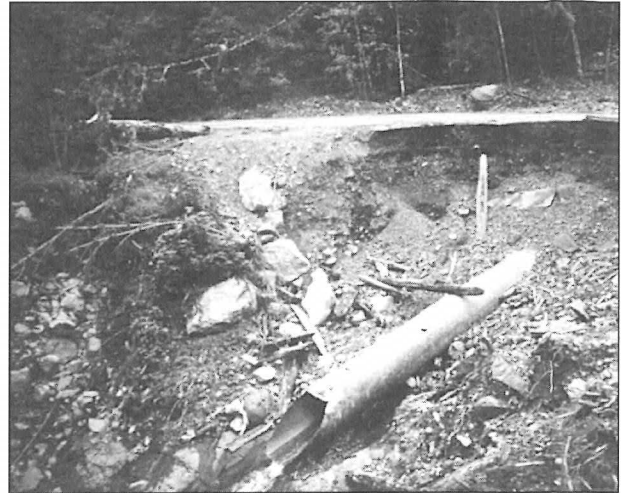
Logging road washout, Second Creek, Mt. Hood National Forest. A debris torrent plugged the culvert, overflowed the road, and continued downstream.
