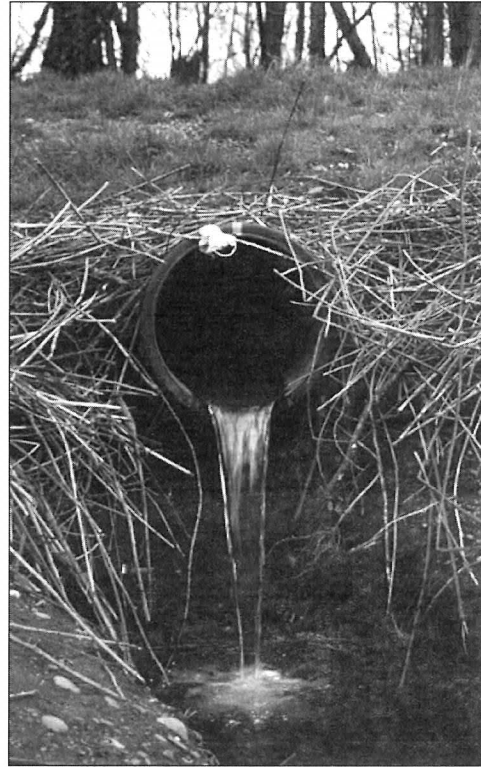
Culverts like this block fish passage into small streams that could otherwise provide spawning and rearing habitat or refuge areas.
